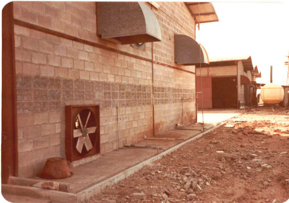
Figure 5.5 Improper Ventilation Design.
