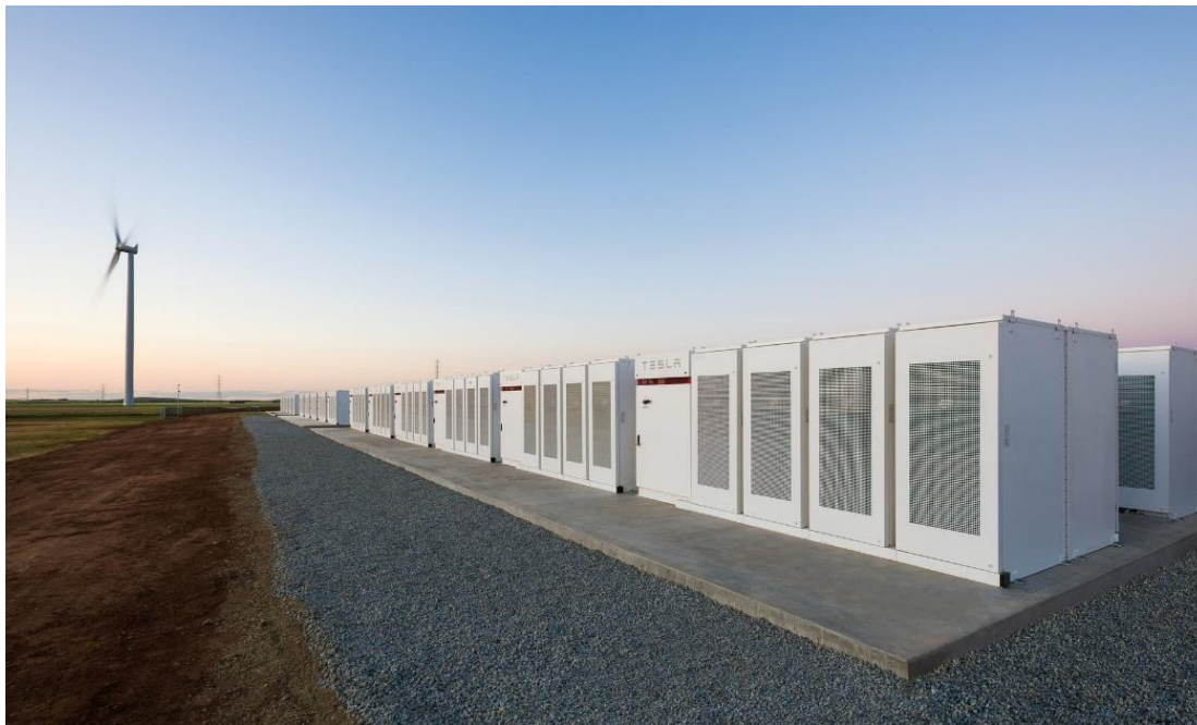
Hornsedale Power Reserve Battery, South Australia
